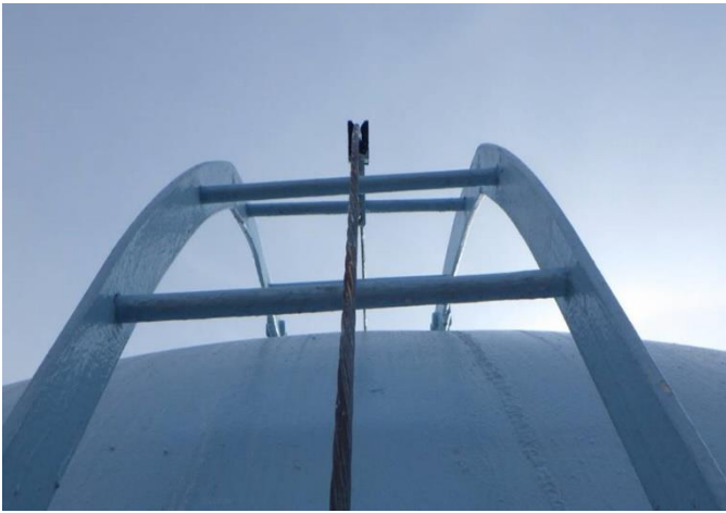
Safety Climb on Access Roof Ladder
