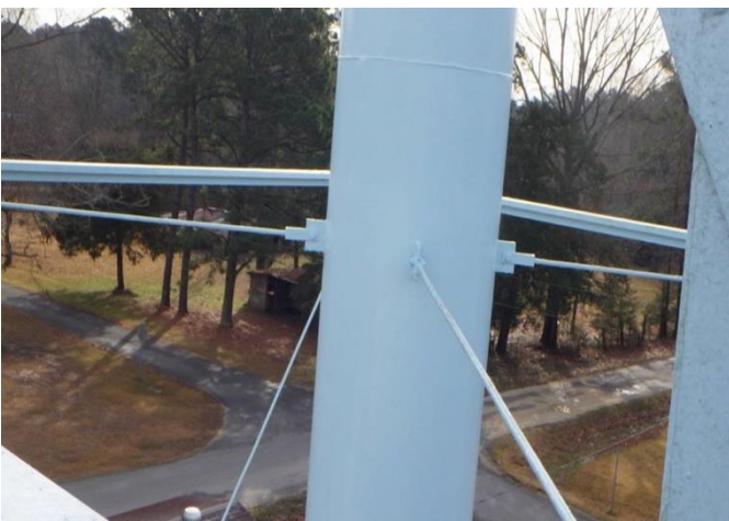
Exterior Coating Riser
