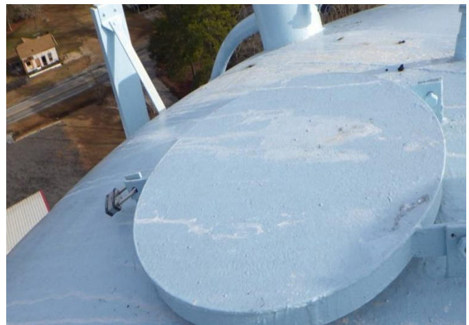
Access Hatch Locked
