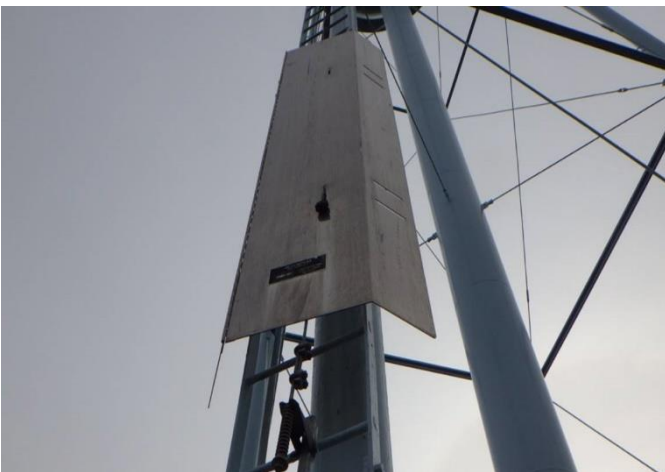
Ladder Guard Locked
