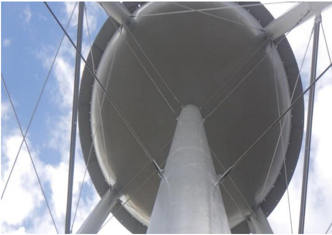
Exterior Coating Under Belly
