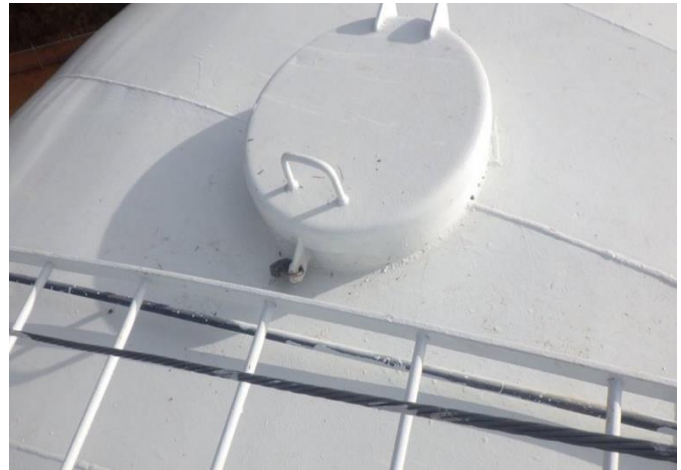
Access Hatch Locked
