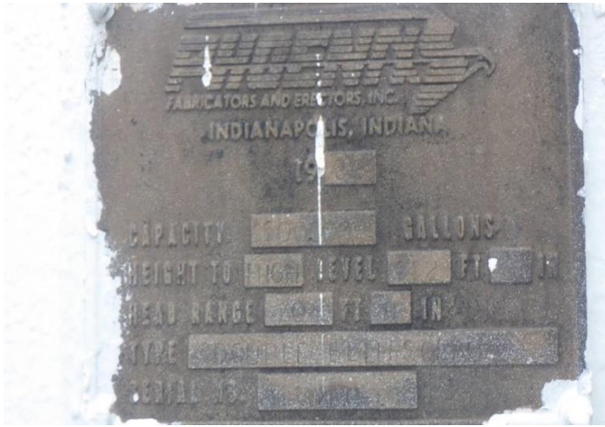
Tank Identification Plate
