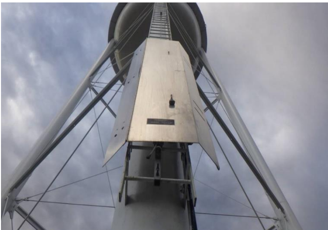
Safety Climb on Access Ladder
