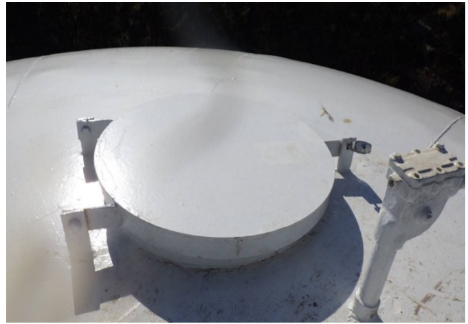
Access Hatch Locked
