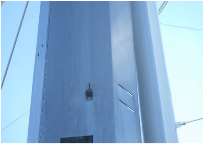
Ladder Guard Locked
